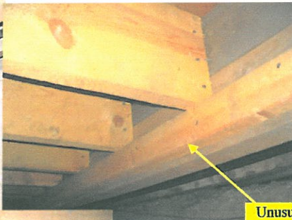
Unusual but apparently sound framing under stacks
