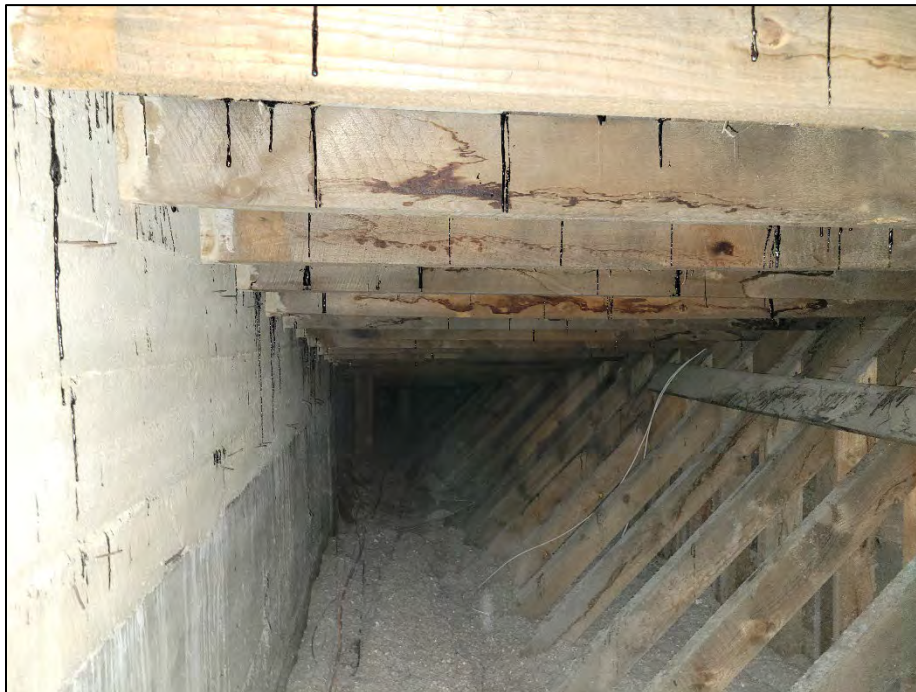
Photo 22. April 11, 2023. First floor storage room: black tar from asphalt roofing on wood ceiling and trusses. Concrete wall. Loose asphalt shingles on floor (off image of photo).
