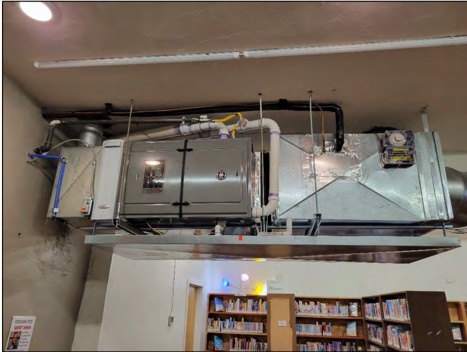
Photo 9. April 11, 2023. Street level. Main library room with modern heating and cooling unit.
