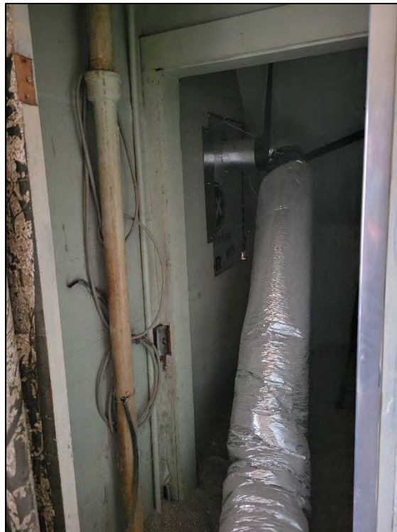
Photo 20. April 11, 2023. First floor, eastern side: utilities and access to attic.
