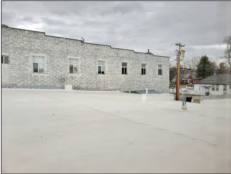
Photo 7. April 10, 2023. Outside on roof. Looking northeast from on the central building roof: Run off drains eastward towards the alley, is collected in gutters, before being discharged into the dirt park area.
