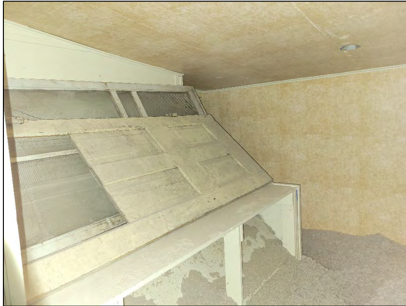
Photo 19. April 11, 2023. First floor: approximately 12 to 18 inches of loose insulation covering the carpeted floor. Multiple doors being stored in room next to bathroom. Wallpaper covering drywall walls and ceiling.
