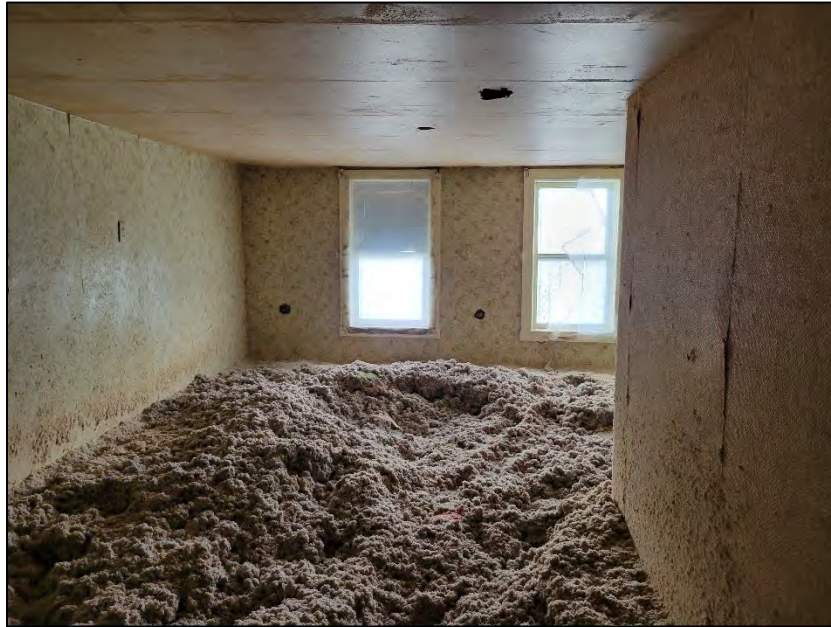
Photo 17. April 11, 2023. First floor: approximately 12 to 18 inches of loose insulation covering the entire upper-level floor. Beneath the insulation is various carpeted flooring. Walls are covered in multiple styles of wallpaper which is covering plaster or drywall walls and ceiling.
