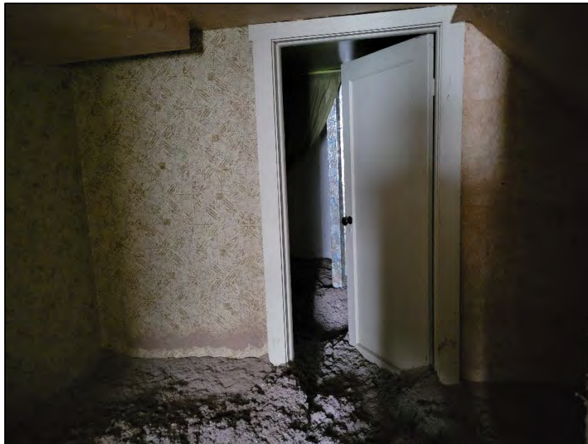
Photo 18. April 11, 2023. First floor: approximately 12 to 18 inches of loose insulation carpeted floors. Upper floor bathroom behind doorway with shower. Multiple types of wallpaper covering drywall walls and ceilings.
