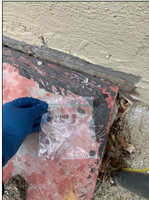
Photo 7. SC18: Silicone / tar between exterior wall (outside of southeastern storage room) and metal lid containing 2% chrysotile ACM. Approximately 2 square feet of surface area.
