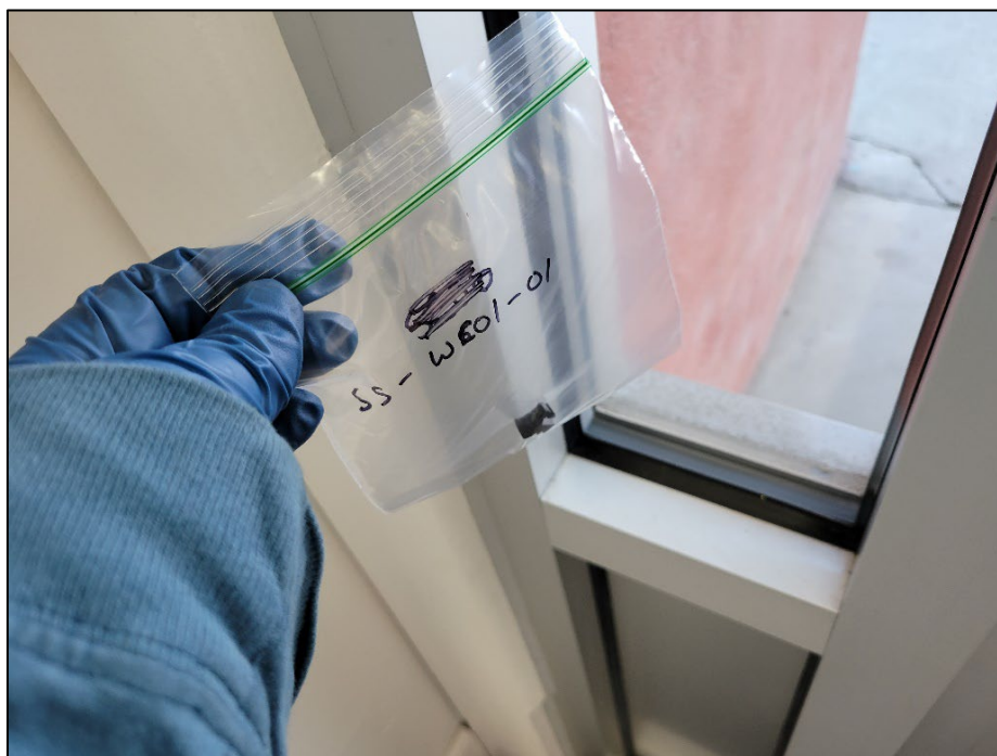
Photo 70. WC01: Window rubber gasket in community room
