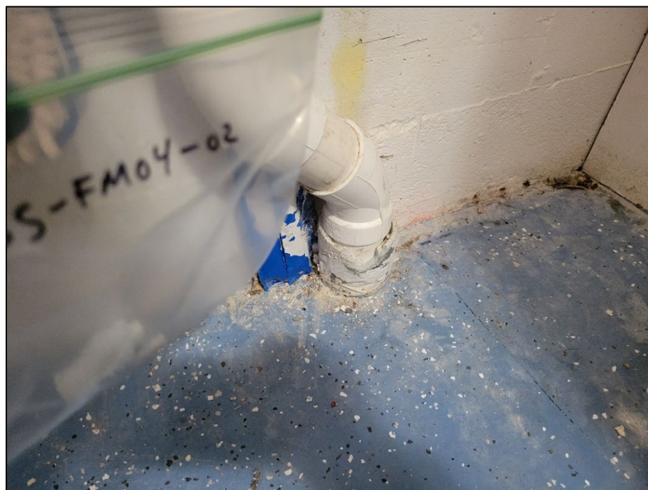
Photo 24. FM04: Silver foam around sewer piping
