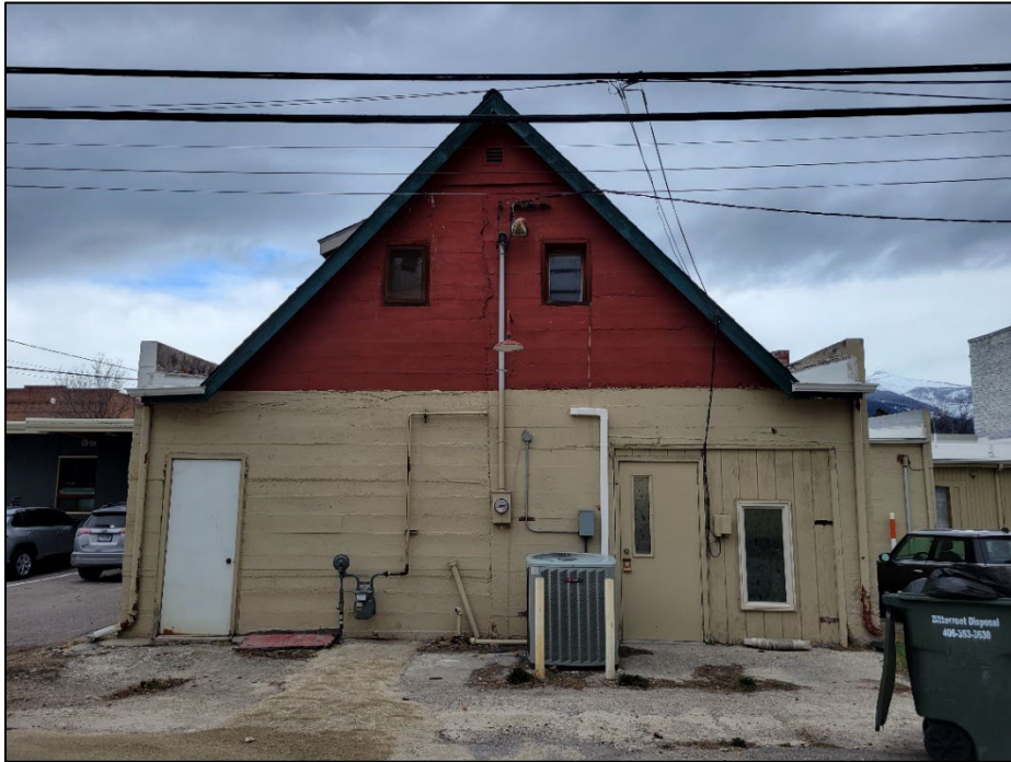
Photo 63. SC19: Black silicone outside of Montana room door
