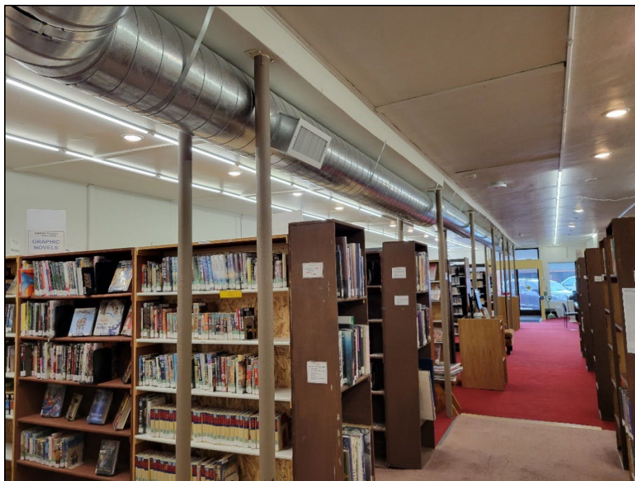
Photo 2. DW02: Drywall ceiling on the southern (left side) of the heating/cooling duct in the main library street level ceiling containing 3% chrysotile ACM. The north side of the duct is plaster (non-detect for ACM).
