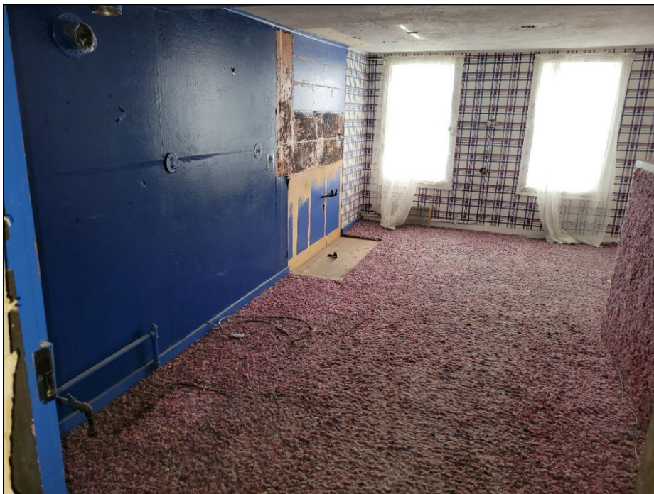
Photo 4. DW02: Drywall ceiling on the first floor containing 3% chrysotile ACM.
