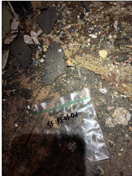
Photo 5. RF01: Asphalt roofing debris on the first-floor storage room containing 7% chrysotile ACM. Approximately 500 square feet of walls and ceiling are present on the first floor, some of which is covered with this debris.
