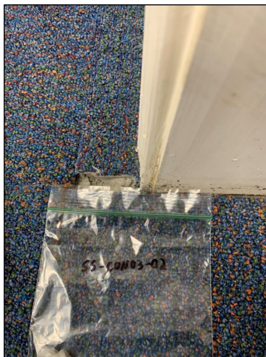
Photo 8. CON03: Concrete under carpet of front desk and community room
