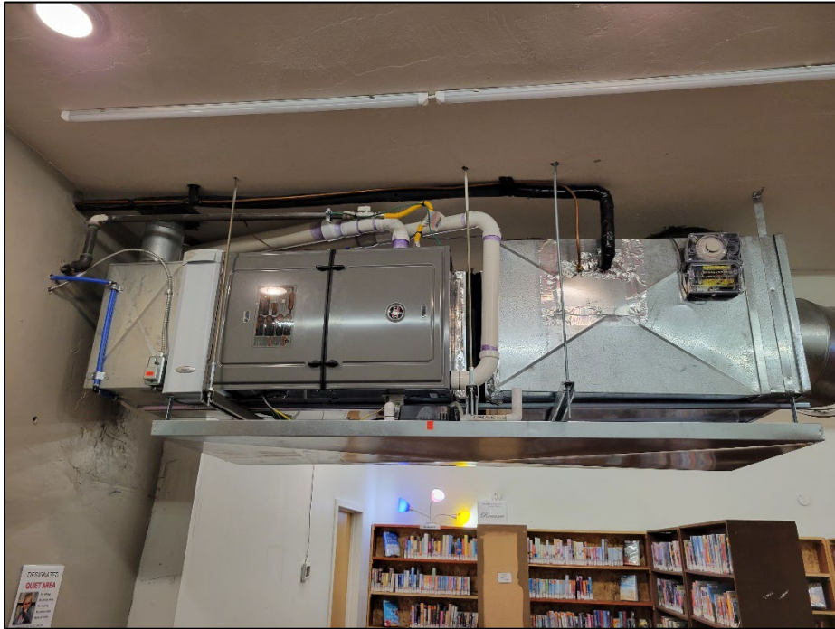
Photo 9. April 11, 2023. Street level. Main library room with modern heating and cooling unit.
