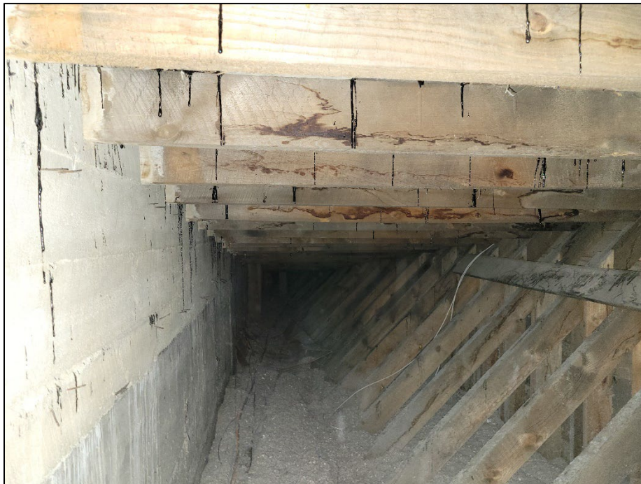
Photo 22. April 11, 2023. First floor storage room: Black tar from asphalt roofing on wood ceiling and trusses. Concrete wall. Loose asphalt shingles on floor (off image of photo).
