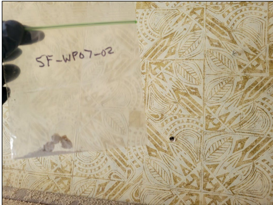
Photo 11. WP07: Drywall behind the wallpaper containing 2% chrysotile ACM. Approximately 7,200 square feet of drywall walls are located on the first floor.
