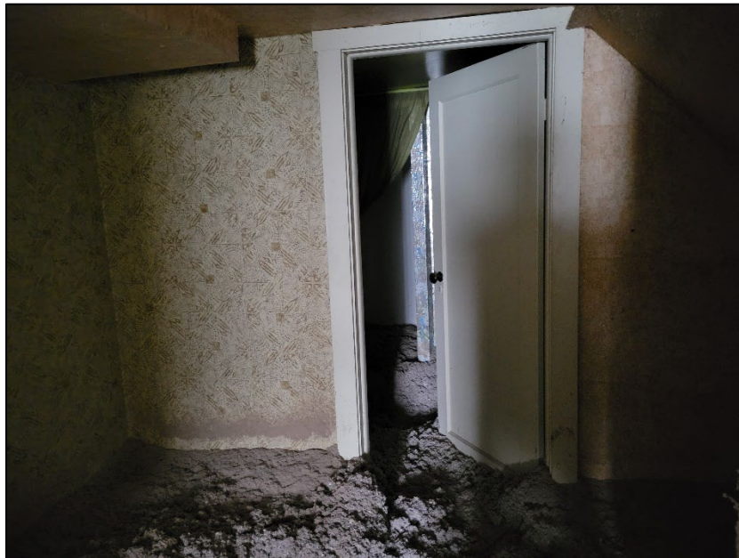
Photo 18. April 11, 2023. First floor: Approximately 12 to 18 inches of loose insulation carpeted floors. Upper floor bathroom behind doorway with shower. Multiple types of wallpaper covering drywall walls and ceilings.
