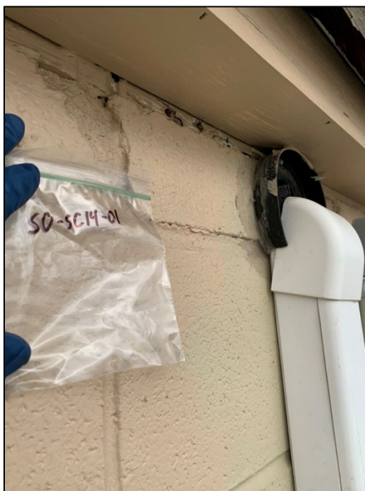
Photo 58. SC14: Silicone outside of in kitchen / staff break room
