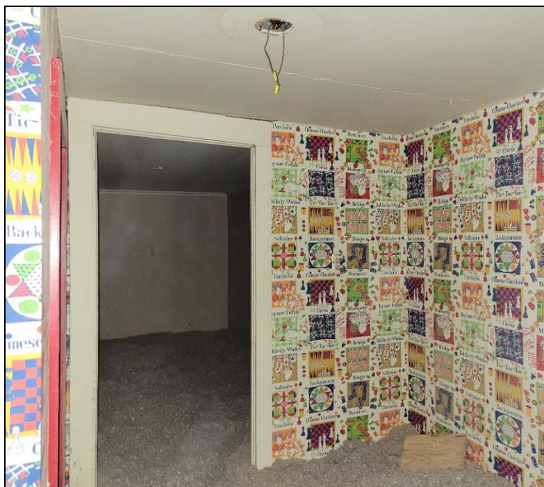
Photo 16. First floor drywall ceiling and walls containing ACM drywall beneath wallpaper. The loose insulation on the first-floor floor is non-detect.
