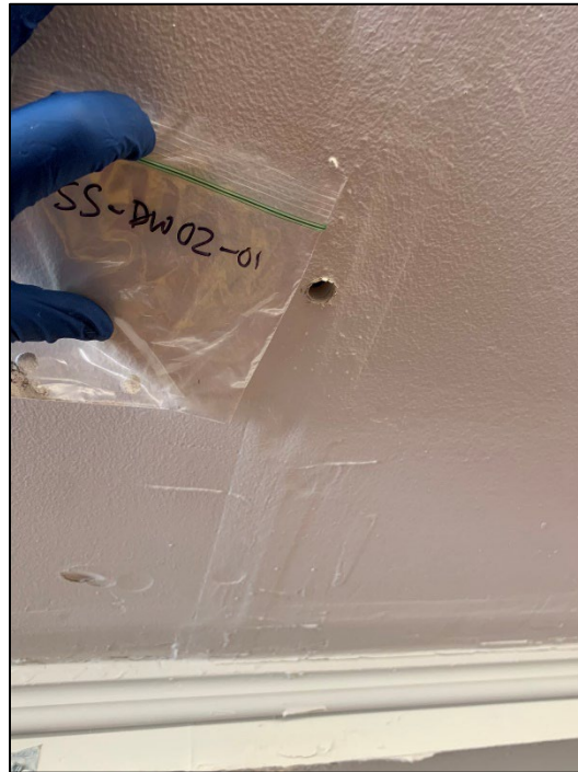
Photo 1. DW02: Drywall (white) containing 3% chrysotile ACM. Approximately, 1,100 square feet of area along the southern side of the main library room ceiling.
