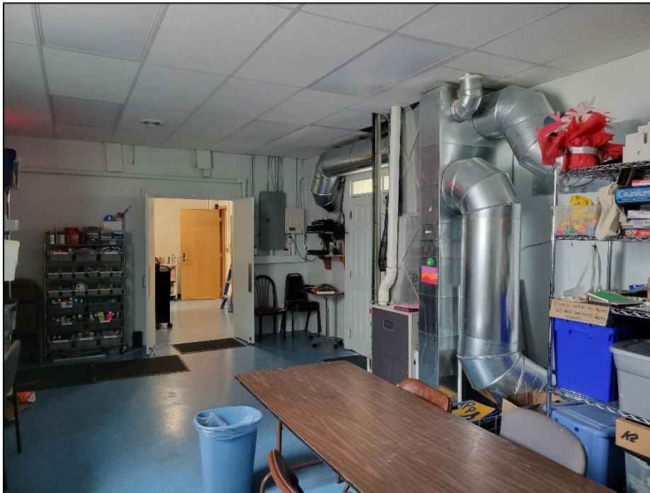
Photo 14. April 11, 2023. Street level. Art room with heating / cooling and breaker box. White painted block and drywall, with similar ceiling tiles to neighboring rooms. Painted concrete flooring. Bathroom are through the central opening where water meter, sewer, and water heater are in bathroom closet.
