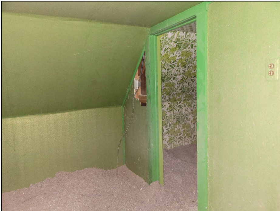
Photo 15. First floor drywall ceiling and walls containing ACM drywall beneath wallpaper. The loose insulation on the first-floor floor is non-detect.
