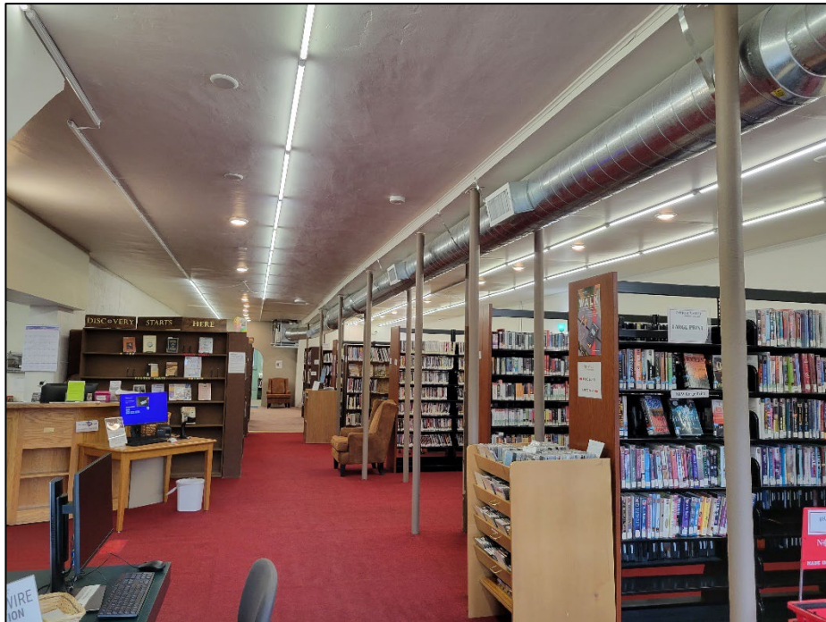
Photo 8. April 11, 2023. Street level. Main library room with white plaster walls / ceiling, multiple carpets covering wood and concrete flooring.
