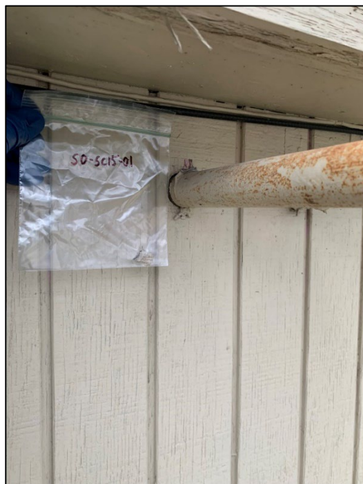
Photo 59. SC15: Silicone outside of furnace / art room
