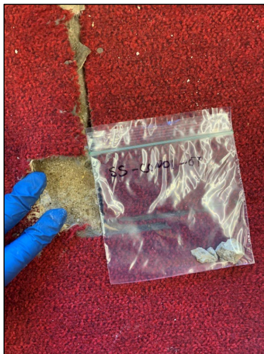
Photo 5. CON01: Concrete under southern half of main library room under red carpet
