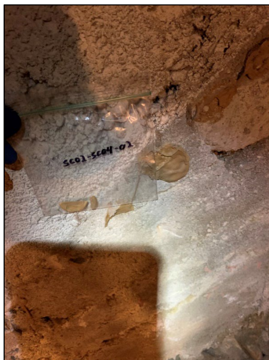
Photo 48. SC04: Silicone in basement under Montana room
