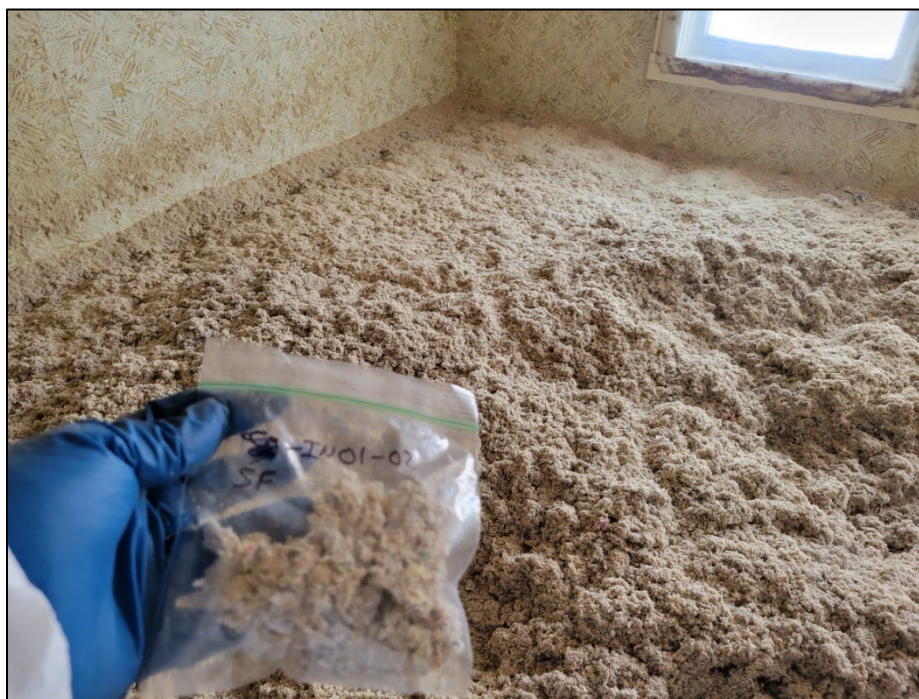
Photo 30. IN01: Loose insulation above Montana room and first floor
