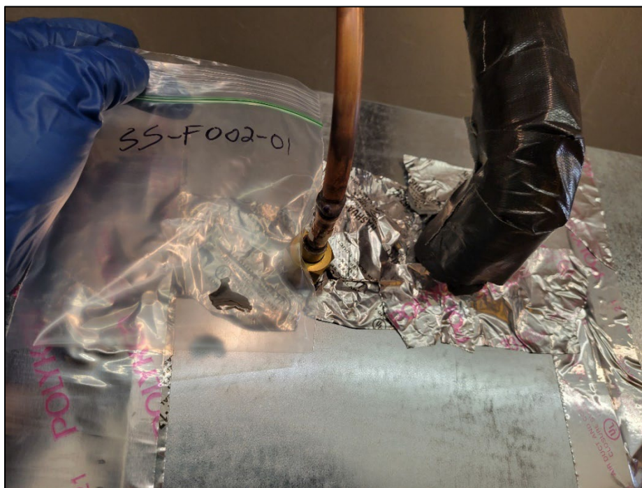
Photo 28. FO02: Black lettering foil on heating/cooling unit near Montana room
