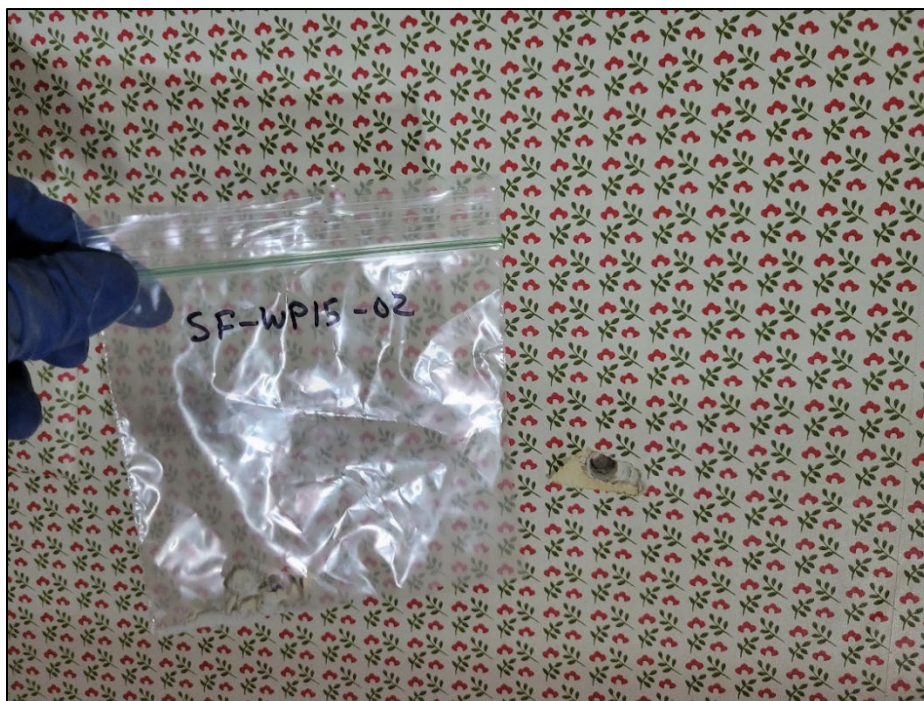
Photo 14. WP15: Drywall behind the wallpaper containing 2% chrysotile ACM. Approximately 7,200 square feet of drywall walls are located on the first floor.
