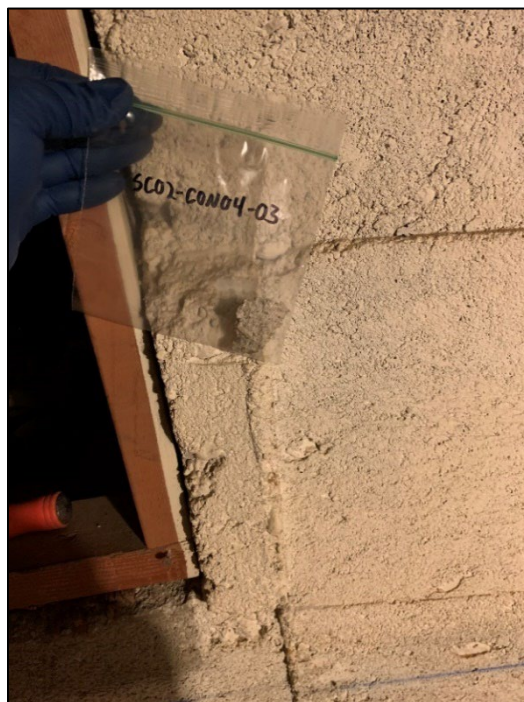
Photo 9. CON04: Concrete under Montana room in basement
