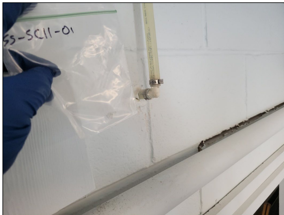
Photo 55. SC11: White silicone in furnace room and bathrooms
