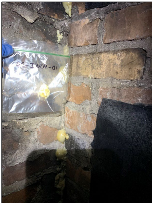
Photo 33. IN04: Spray insulation in basement under front desk
