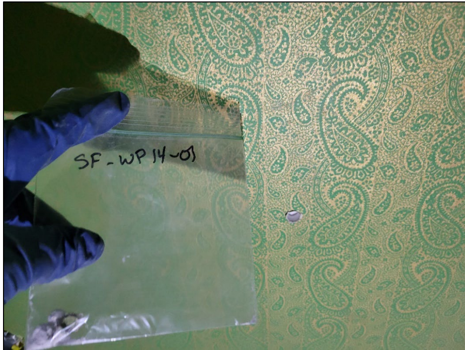
Photo 13. WP14: Drywall behind the wallpaper containing 2% chrysotile ACM. Approximately 7,200 square feet of drywall walls are located on the first floor.
