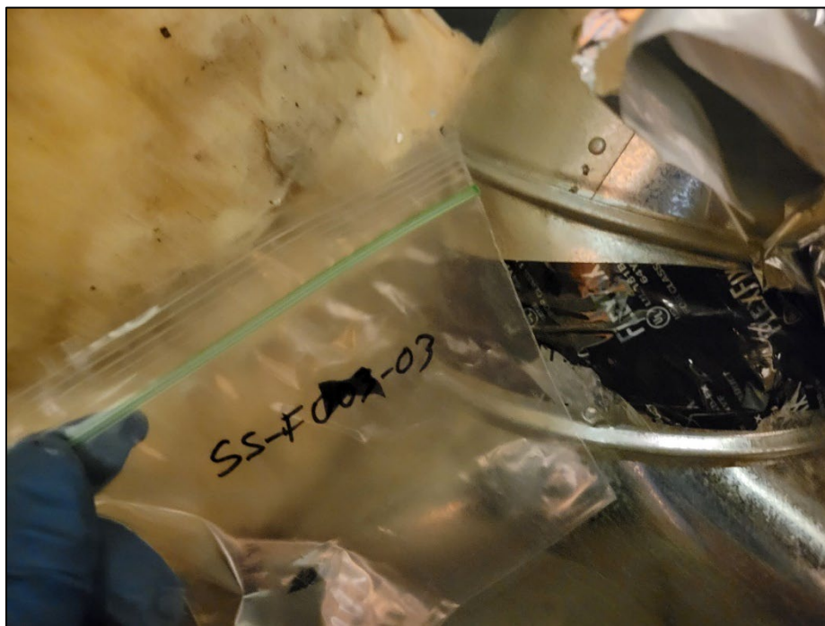
Photo 29. F003: Black foil on heating/cooling piping unit near Montana room
