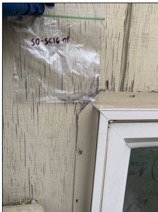
Photo 60. SC15: Silicone outside of Montana room
