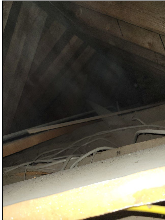
Photo 21. April 11, 2023. First Floor attic: Wood framed attic with loose insulation, black tar from roof, and utilities running over trusses.
