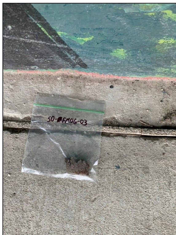
Photo 26. FM06: Expansion foam outside of main library entrance
