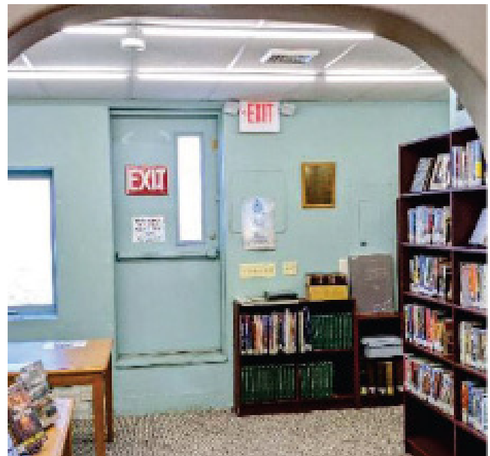
Figure 9: 17-inch step up is not ADA accessible
